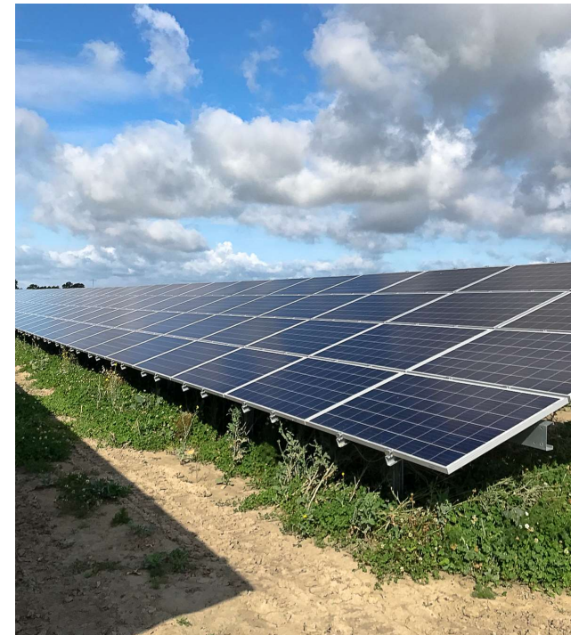
Better Energy, Denmark: 60MW over multiple projects
